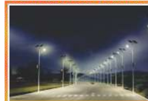
Road & Street Lights
